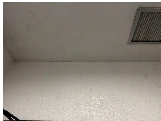
(d) Damage to the infill wall and plasterboard ceiling joint
