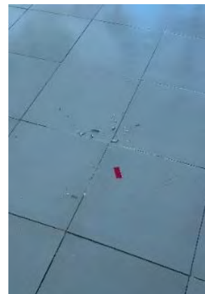
(d) Damage to ceramic tile floor covering
