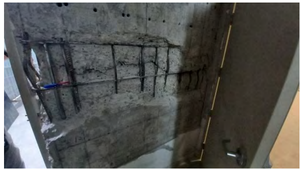
(d) Through-thickness failure of short wall in X-direction with repair initiated, looking from inside
