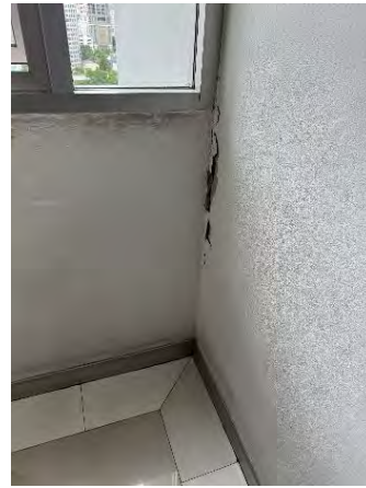
(f) Damage to infill wall joints
