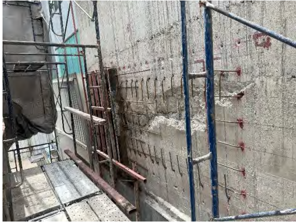
(i) Damage to Y-dir wall on the perimeter (next to stair), wall under repair
