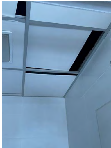
(a) Damage to grid-and-tile ceiling on Floor 18 of Building H1
