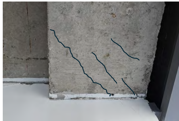
(c) Cracking on soffit of beam (crack width ~0.2 mm)
