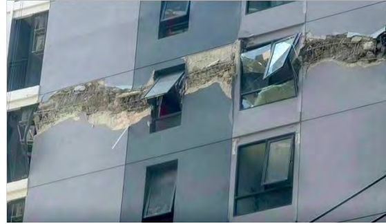
(b) Wall damage on the 9 th floor
