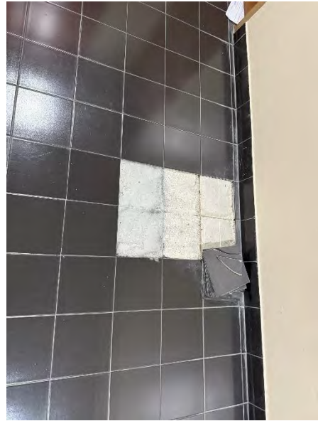
(f) Tile spalling
