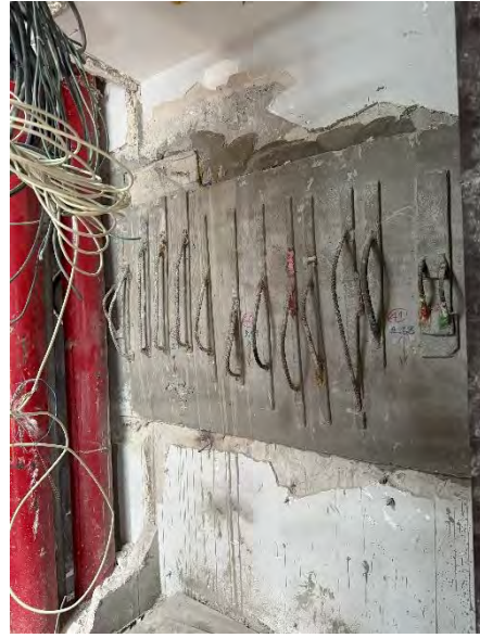
(j) Buckled rebar in stair well
