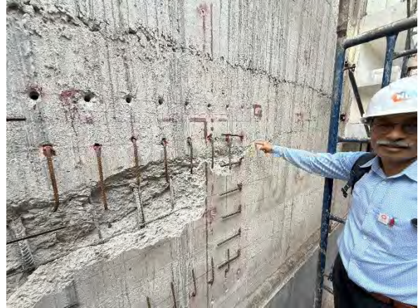
(j) Damage along cold joint
