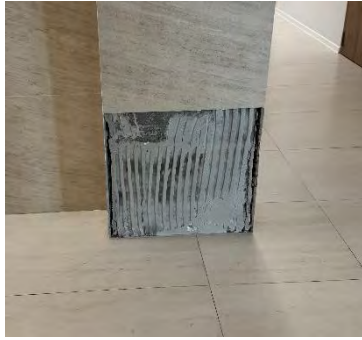
(e) Falling of granite tile (Storey 18)
