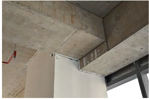
(b) Joint at beam and slab damage
