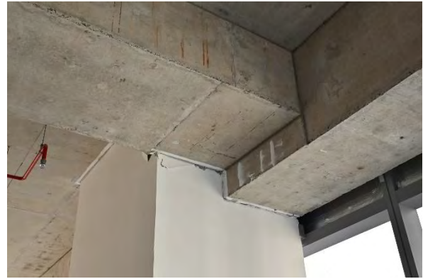
(b) Joint at beam and slab damage
