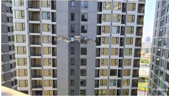
(a) Wall damage on the 9 th floor
