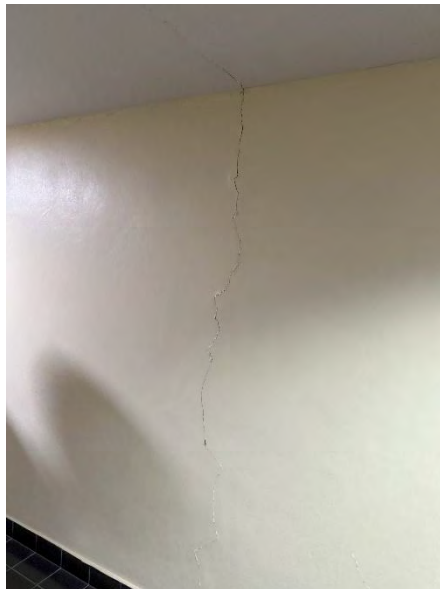
(g) Cracking to wall and ceiling
