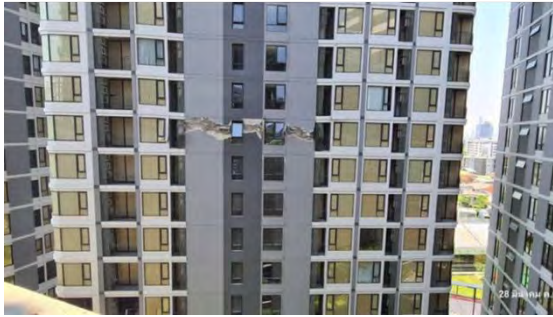
(a) Wall damage on 9 th floor
