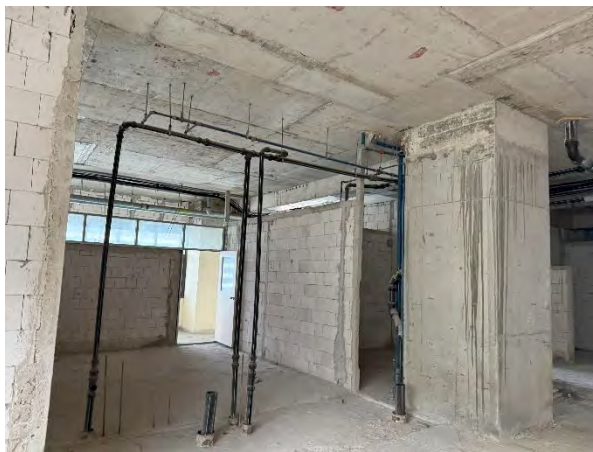
(c) Services pipes layout, note no bracings
