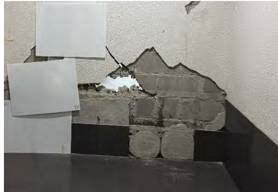
(f) Damage to infill wall (Story 17).
