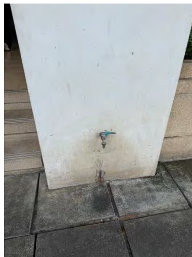
(b) Damage to water supply tap on Floor 5 of Building R3
