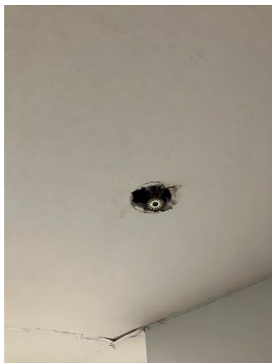
(a) Ejection of sprinkler escutcheon on Floor 18 of Building H1
