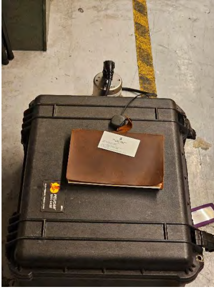
(a) Photo of Station 01 in the storage room on Floor 76
