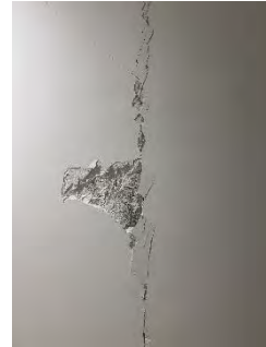
(b) Damage to infill wall (Storey 14)
