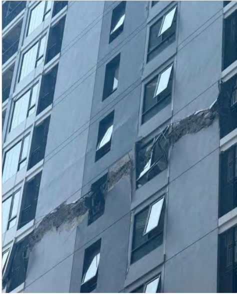
(c) Wall damage on the 9 th floor
