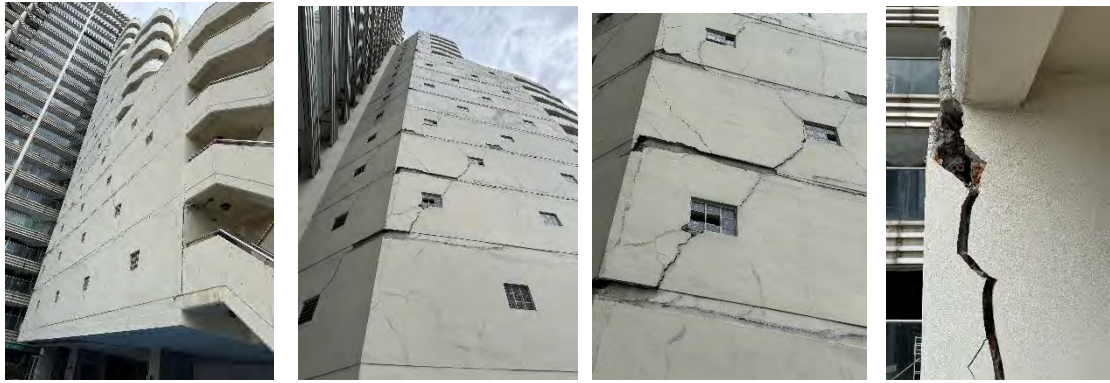
(a) Damage to exterior clay brick wall as seen from outside
