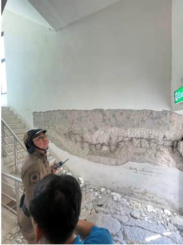
(a) Through-thickness failure of the wall along gridline Y9
