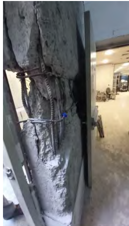
(c) Through-thickness failure of the wall in the X-direction
