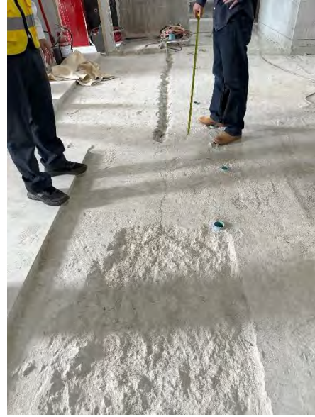
(f) Damage to the floor
