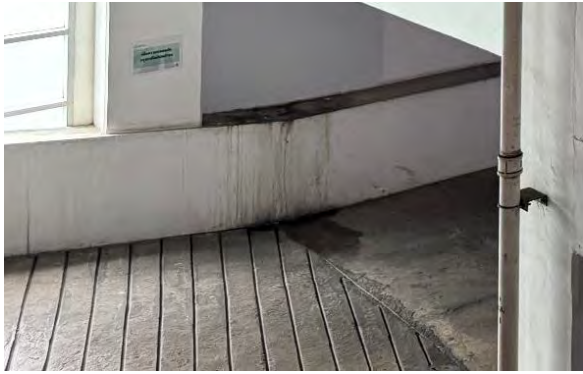
(c) Location of water leakage from the surge tanks of swimming pools due to joint cracks (Floor 5A)
