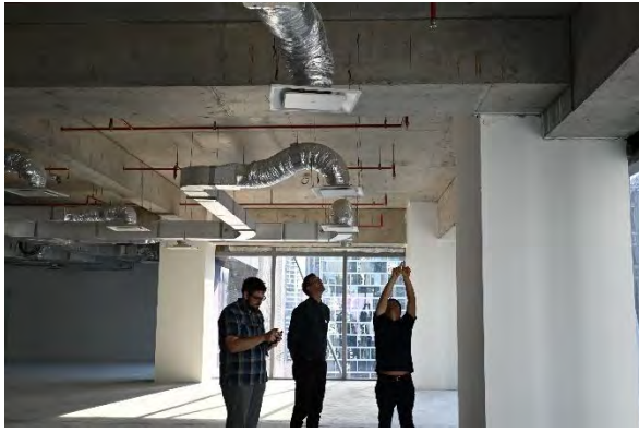
(a) Location of beam and ceiling slab damage
