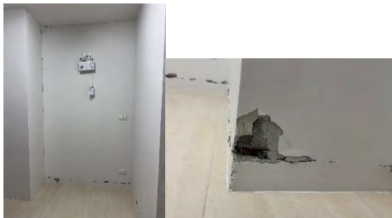
(a) Damage to infill wall (Storey 18)
