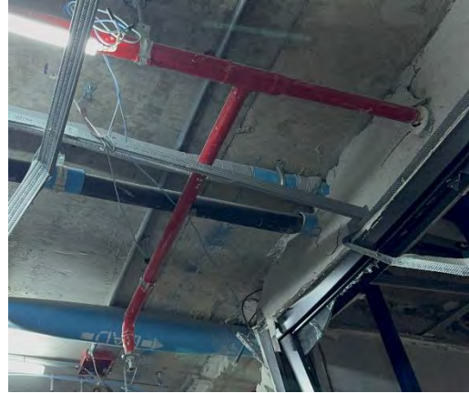
(d) Damage to infill walls due to interaction between pipes and wall, 9 th storey
