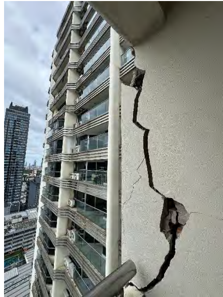
(b) Severe cracking to the stairwell and masonry partitions
