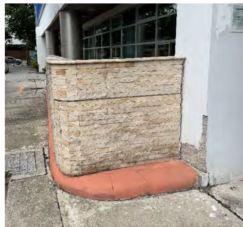
(b) Damage to short boundary wall (Ground Floor)
