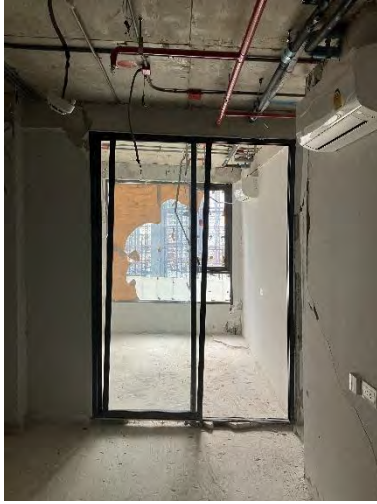
(c) Damage to glass door frames, 9 th storey
