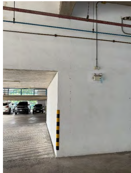
(h) Cracking at the interface of the structural and non-structural wall
