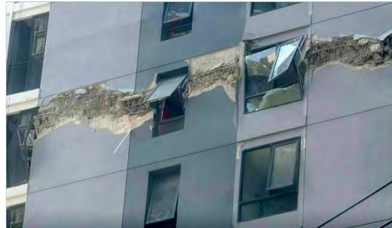
(b) Wall damage on 9 th floor
