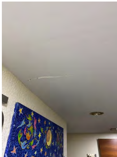
(b) Damage ceiling on Floor 15 of Building R2
