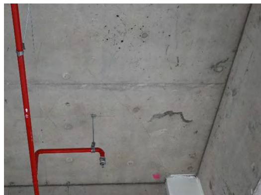
(e) Cracking on the soffit of the floor slab by the beam exterior beam-column joint (crack width ~0.3 mm)
