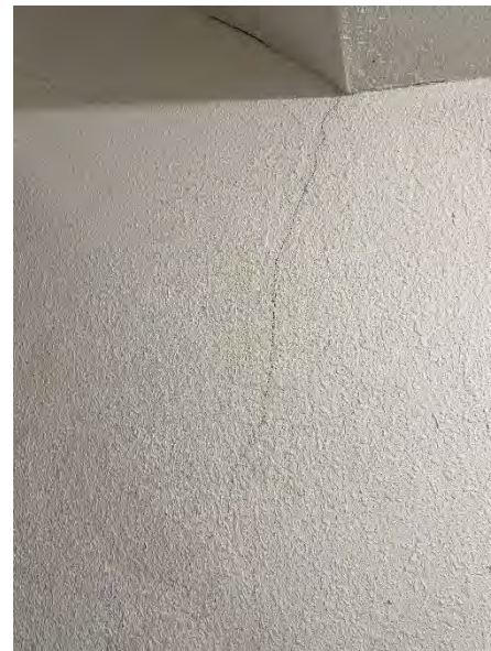
(h) Cracking damage at the interface of infill and structural wall.
