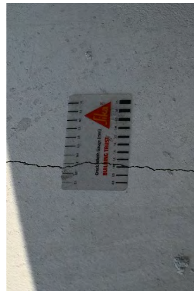
(e) Measurement of floor topping crack (crack width = 1.0 mm)
