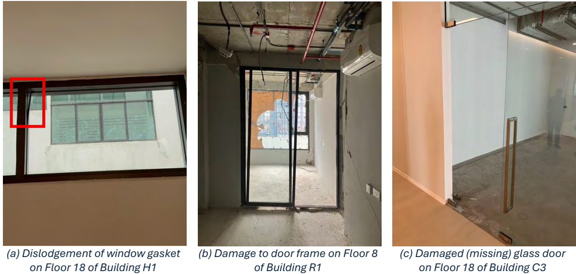
Figure 22: Photos of typical damage to doors and windows
