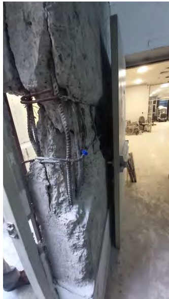
(c) Through-thickness failure of the wall in the north-south direction
