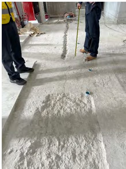
Figure 32: Cracking to the floor in Building R1
