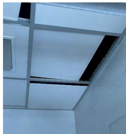
(f) Ceiling tile dislodgement
