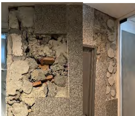
(c) Damage to granite tiles on core walls (Story 20)
