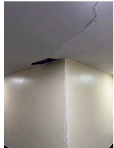
(b) Damage ceiling on Floor 18 of Building R2
