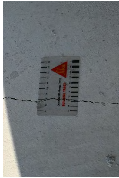
(g) Measurement of floor topping crack (crack width = 1.0 mm)
