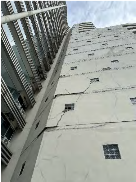
(a) Moderate cracking around the perimeter of the exterior masonry partition wall
