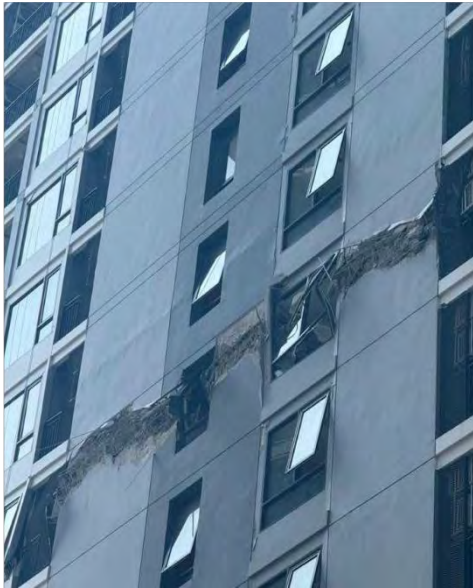
(c) Wall damage on 9 th floor
