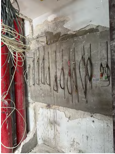
(i) Buckled rebar in stair well
