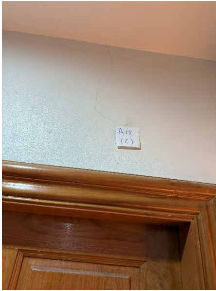
Figure 42: Cracking to non-structural wall in Building R4.
