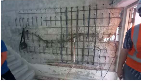
(a) Repair to through-thickness failure of wall in y-direction
