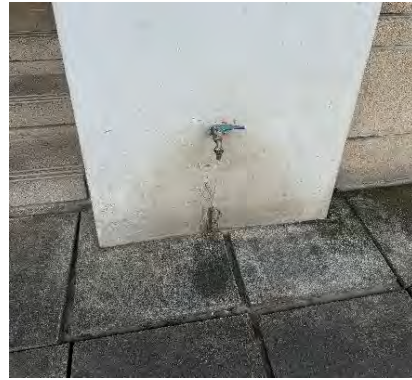
(d) Damage to the water pipe and water shut off to the tab (Floor 6)
