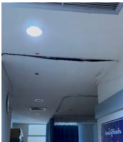
(e) Damage to plasterboard ceiling
