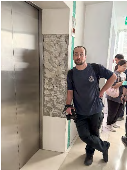
(g) Tile spalling
