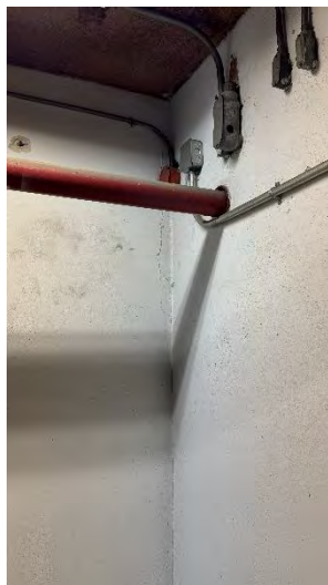
(a) Damage to infill wall (Story 34)
