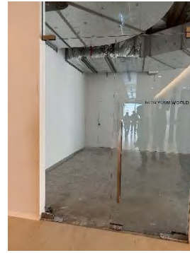
(f) Damage to the glass door (Storey 18)
