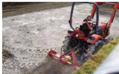
A small tractor and rotovator attachment used to mix cement with soil
