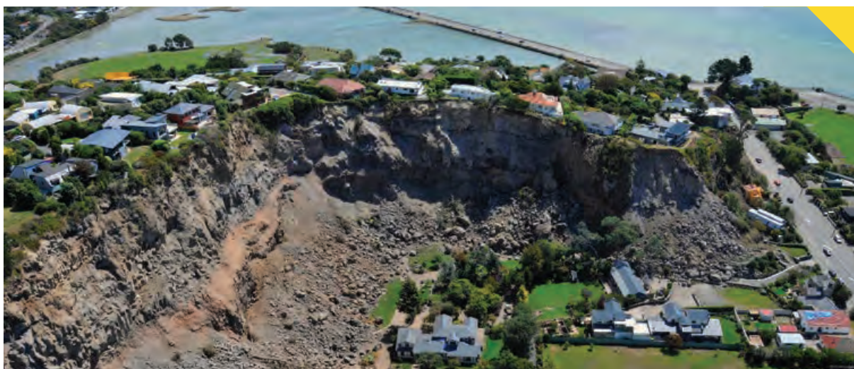
► Rockfalls on cliffs, Redcliffs following Christchurch earthquakes 2011. Photo: Graham Hancox
