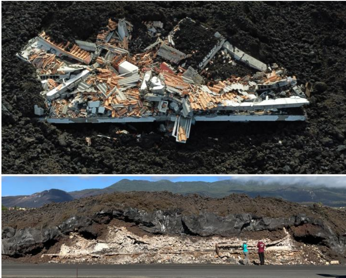
Figure 11. Complete damage to houses and other buildings as examples of Damage State 5 within the lava flow field.
