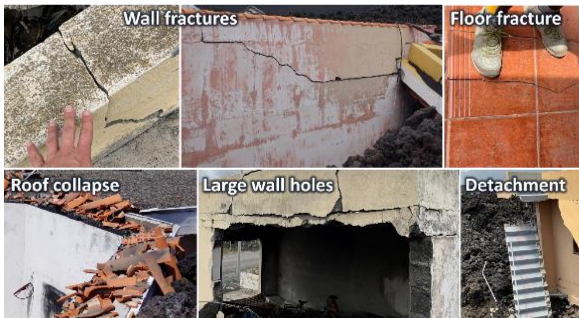
Figure 7. Examples of damage caused by lateral load, or pushing by the lava flows.
