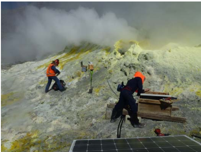
Fig. 1. F0 site on White Island. Elemental sulfur forms the chimney around the vents, and the area where the installation will reside is periodically bathed in emissions, hence the requirement for effective protection from the corrosive gases.
