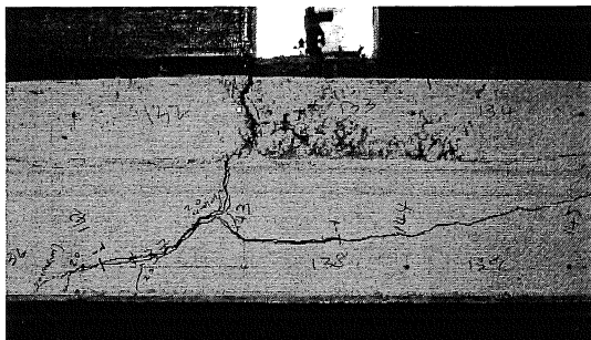
(i) Shear crack at -2.0% drift at northern side
