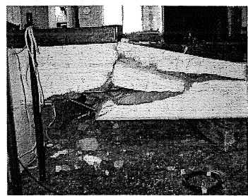
(iii) Connection at failure
