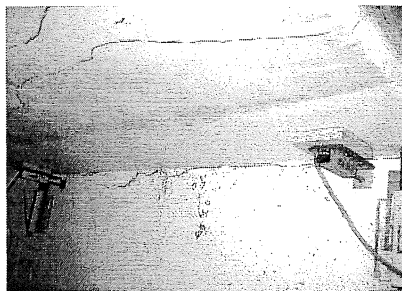
(i) Cracks at the underside of the unit at 1.0%
