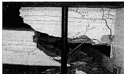
(ii) Unit being hang on by strand at failure
