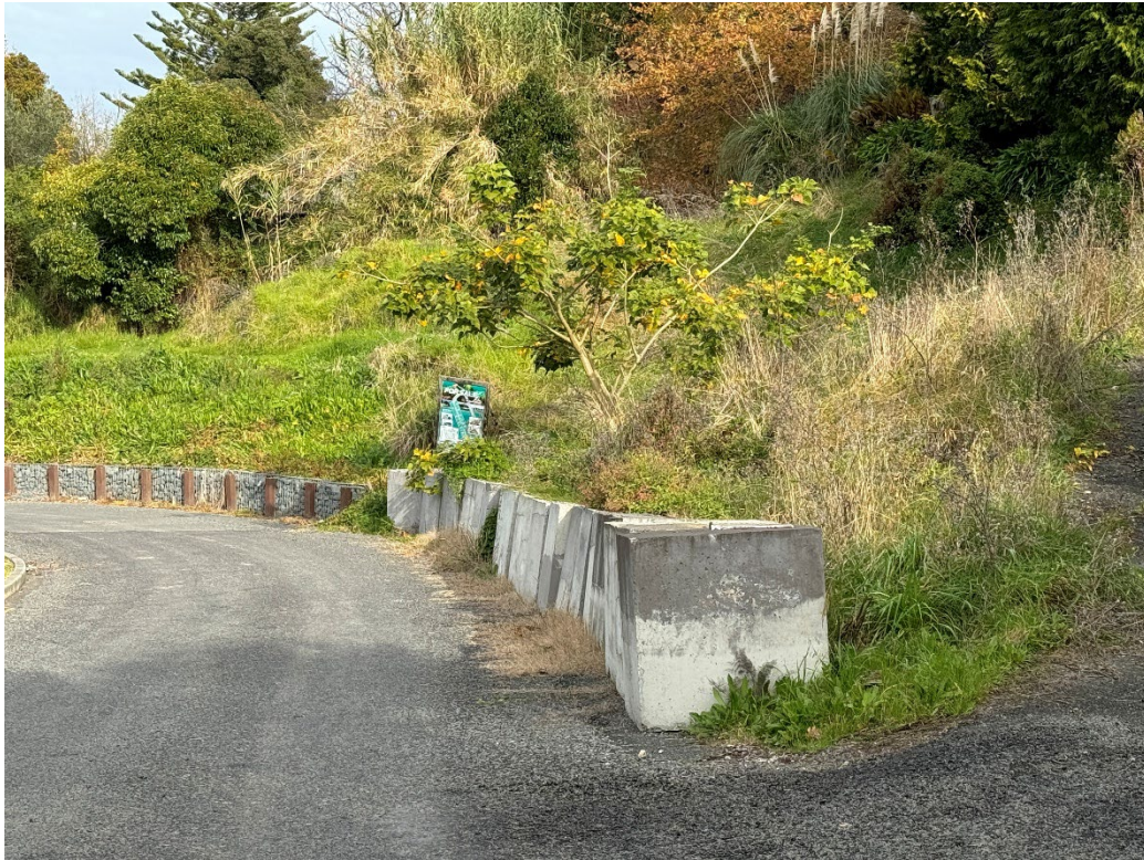
Figure 13: Retaining blocks (1 m high) at toe of Russell St landslide, showing evidence of uplift (heave).
