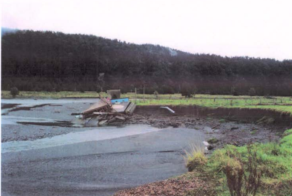
Fig. 10 New milking shed undermined by river eroding into valley-side fan deposit 3 years after dambreak
