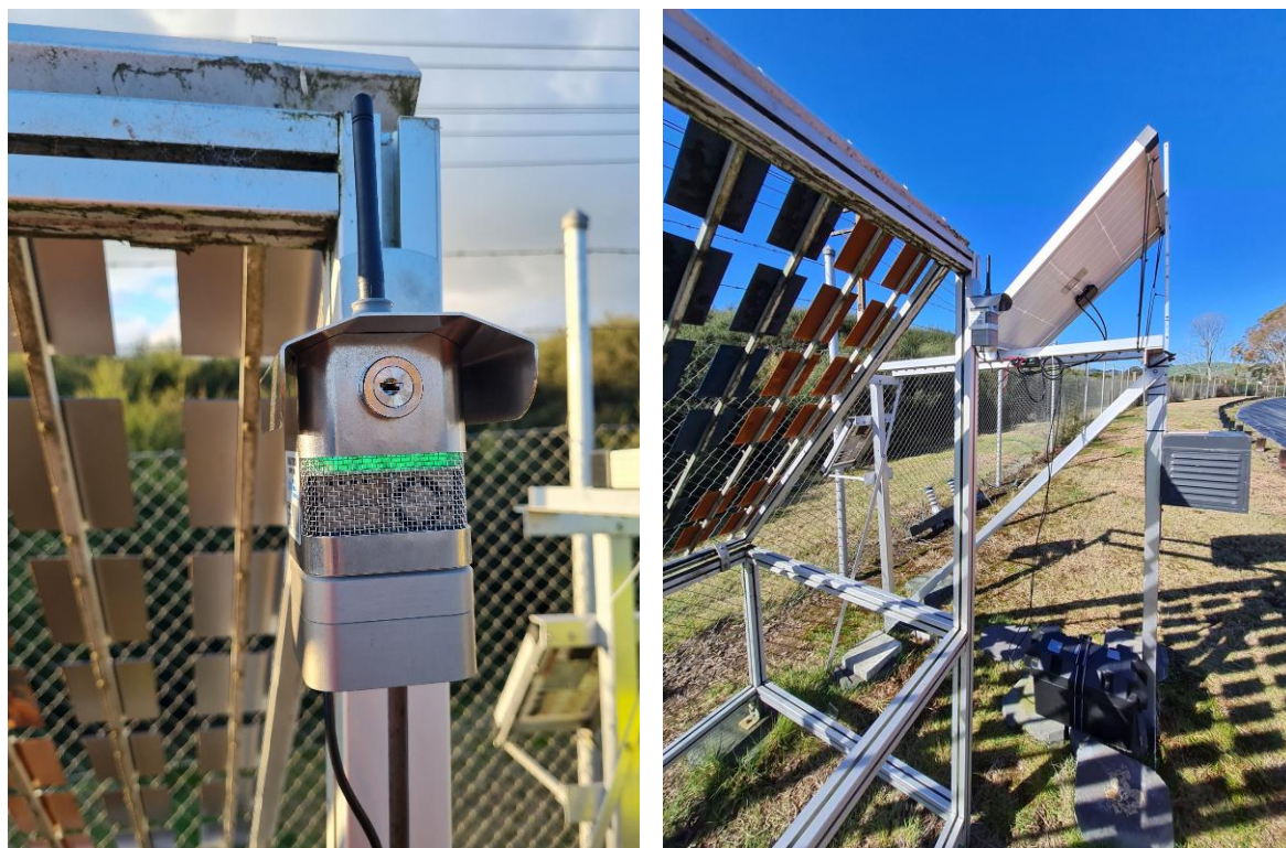
Figure 6 Air quality sensor installed at wastewater treatment plant site. (a) Airly sensor and (b) solar array.
