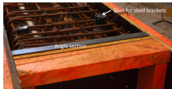
(c) Duct at column base for attaching steel bracket to column face
