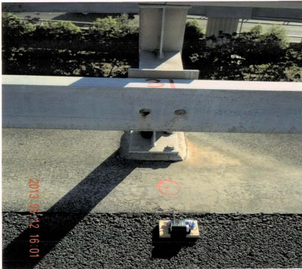
Figure 6.12. USB accelerometer installed on the bridge deck.
