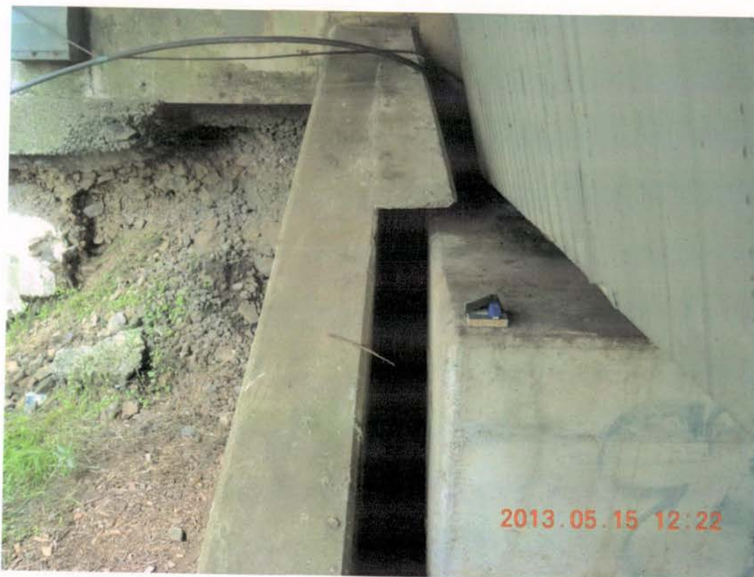
Figure 6.14. USB accelerometer installed on bridge abutment.
