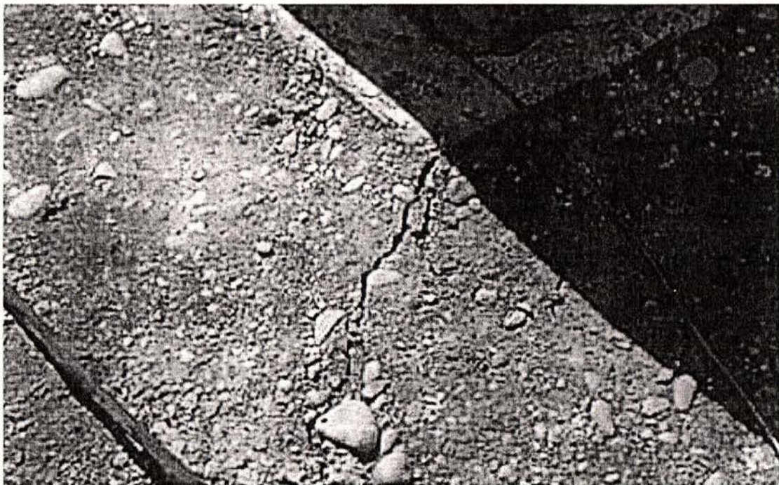
Figure 4.17. Cracking in the soil, running diagonally away from the foundation beam edge closest to the reaction pile cap.
