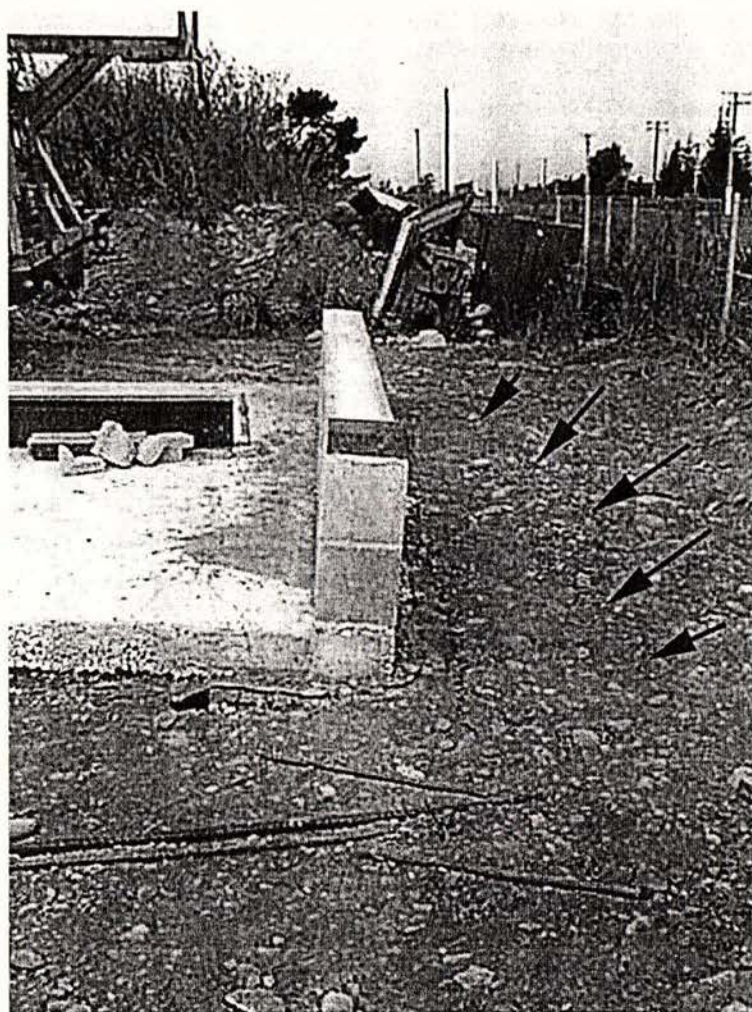
Figure 4.11. Rotation of the foundation beam, masonry wall, and part of slab furthest from the reaction pile cap.
