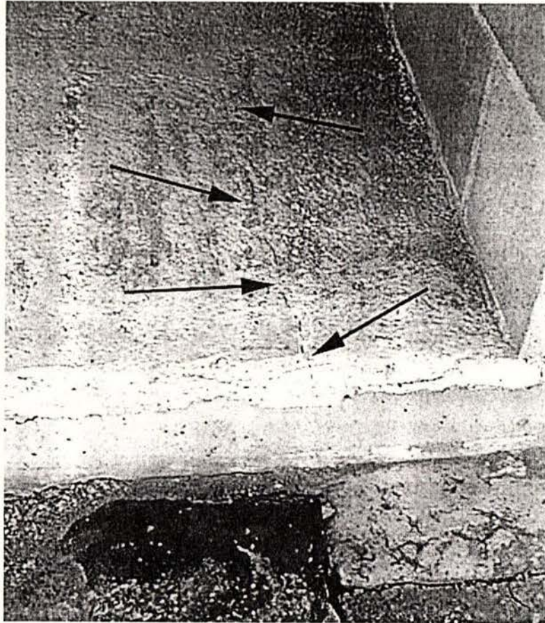
Figure 4.15 Arrows show cracking in the top of the slab during load step 2.
