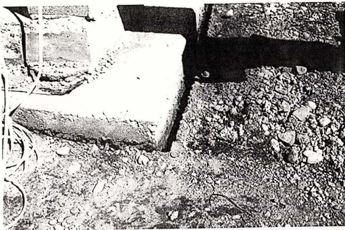
Figure 4.2. Uplift of foundation beam, load step 1.
