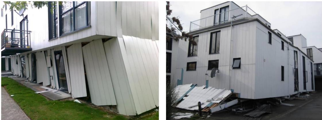
Figure 13. Soft storey collapse of ground floor observed in the canterbury earthquake sequence
