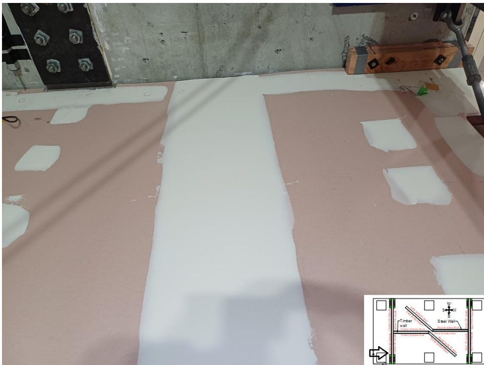
Figure 2.65. Timber Southeast Outside wall after motion 18 - 3 % inter-storey drift
