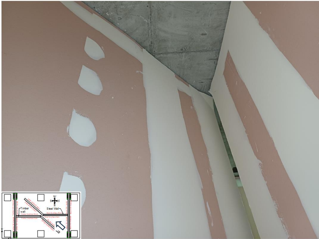
Figure 2.70. Timber wall inclined junction West and Steel wall inclined junction East after motion 18 - 3 % inter-storey drift
