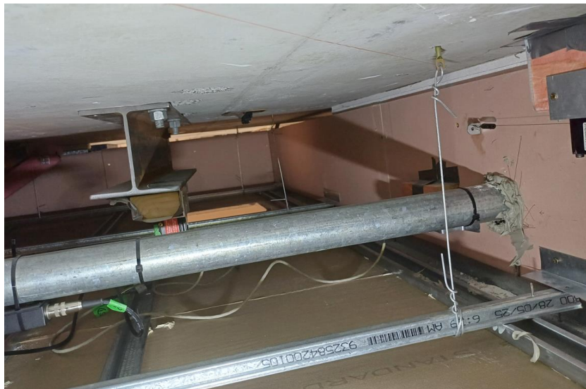
Figure 3.20. Photo of constructed specimen inside the ceiling plenum
