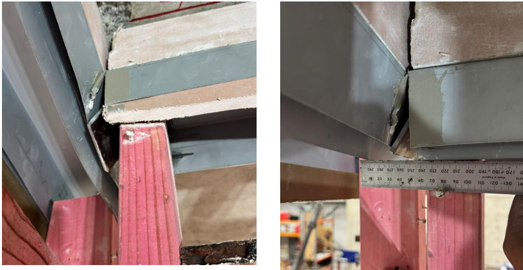
Figure 4.68. Photo of bent top steel angle at North wall junction taken during demolition
