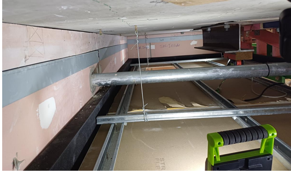
Figure 4.16. Photo of constructed specimen inside the ceiling plenum
