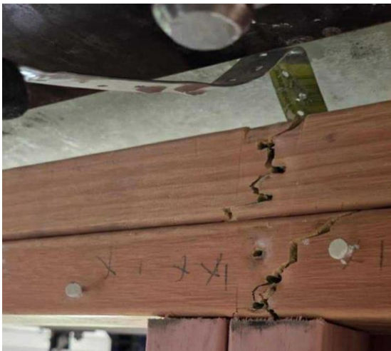
Crack in the top plate
