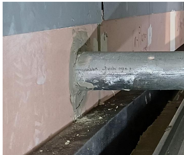
b) Pipe penetrating through wall with fire-sealant applied
