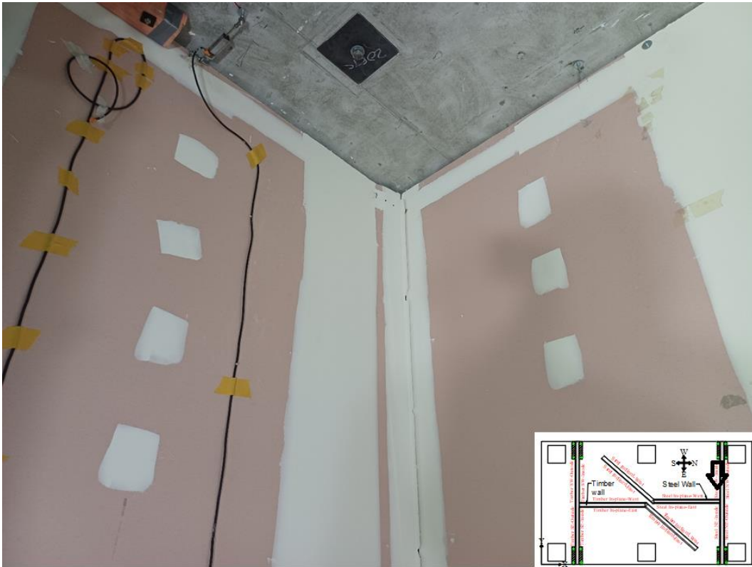
Figure 2.58. Steel wall west return junction after motion 18 - 3 % inter-storey drift
